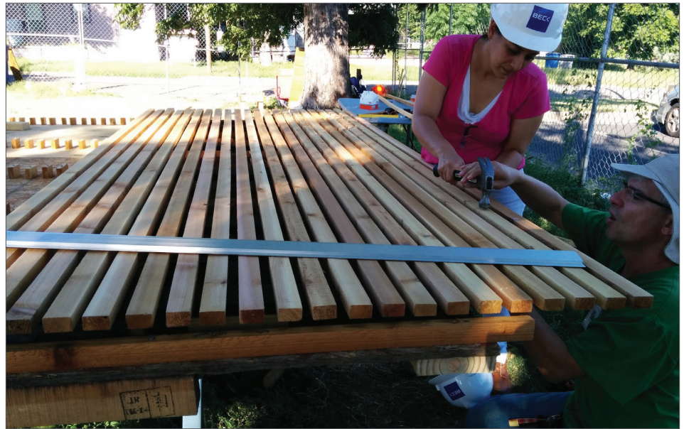
Fig. 01 Quality control on rainscreen ensuring the proper installation of screws placed trough jig.
