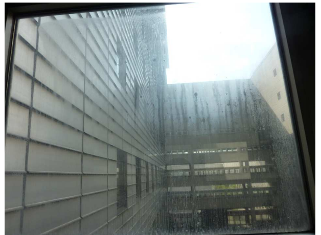
Fig. 10 Condensation on windows show that the indoor air quality is too cold and humid compared to the outdoors.
